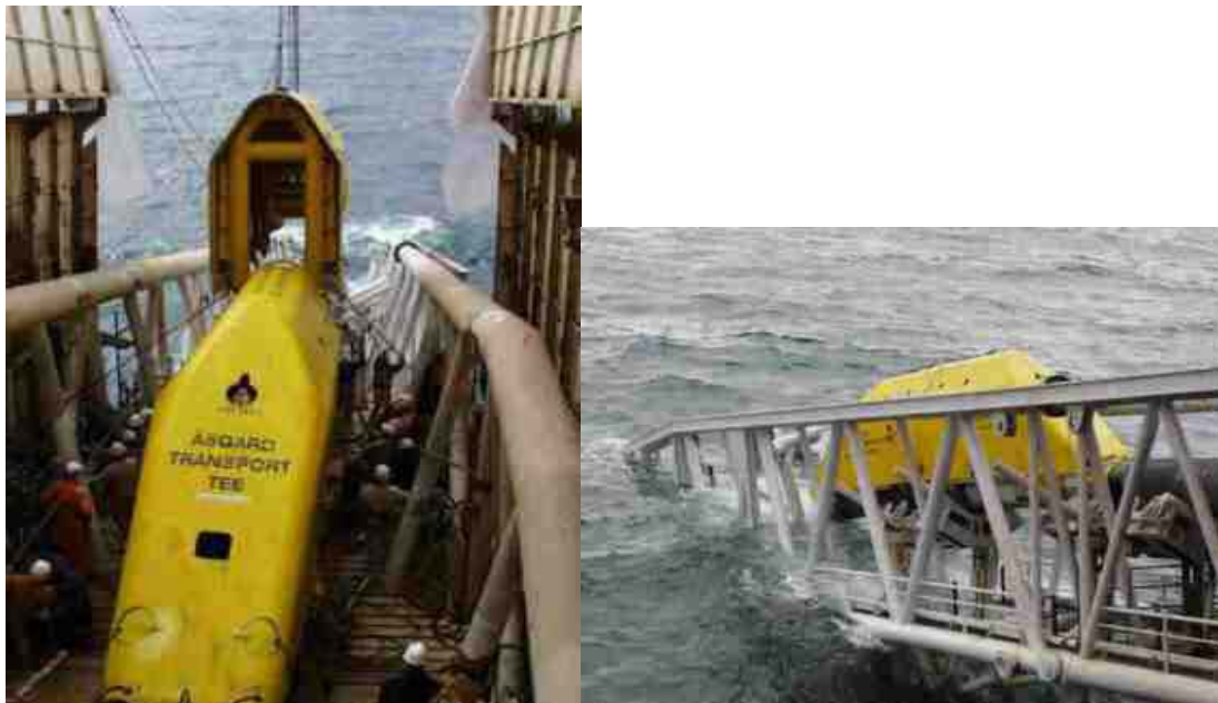
Two 8m GRP covers landed over steel frames attached to the pipeline at the lay barge.
